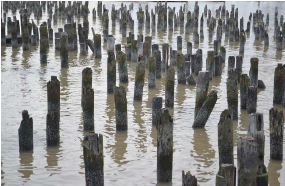
Decaying piers near Pier 59
