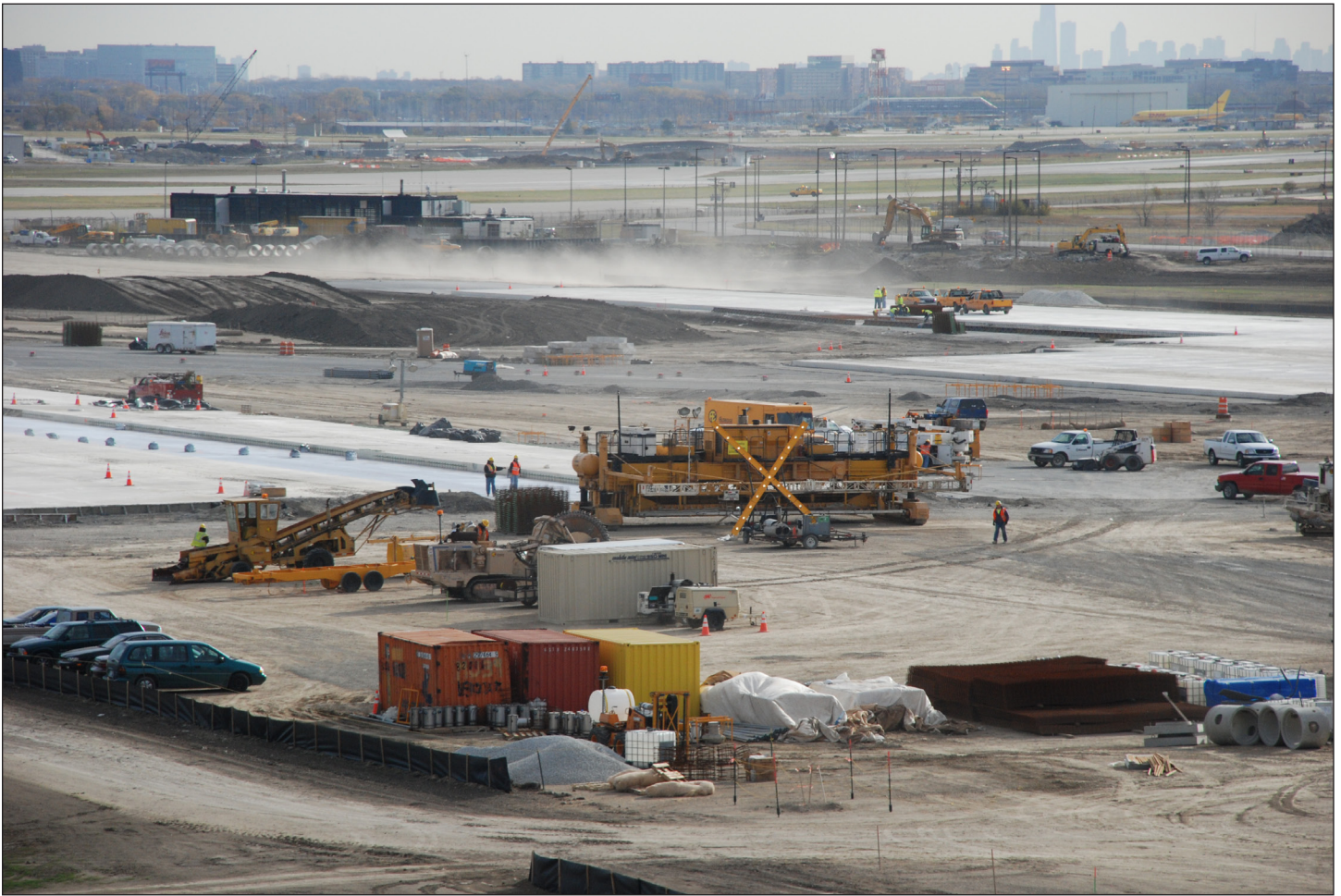
Runway construction at Chicago O'Hare International Airport (photo courtesy of the Chicago Department of Aviation).
