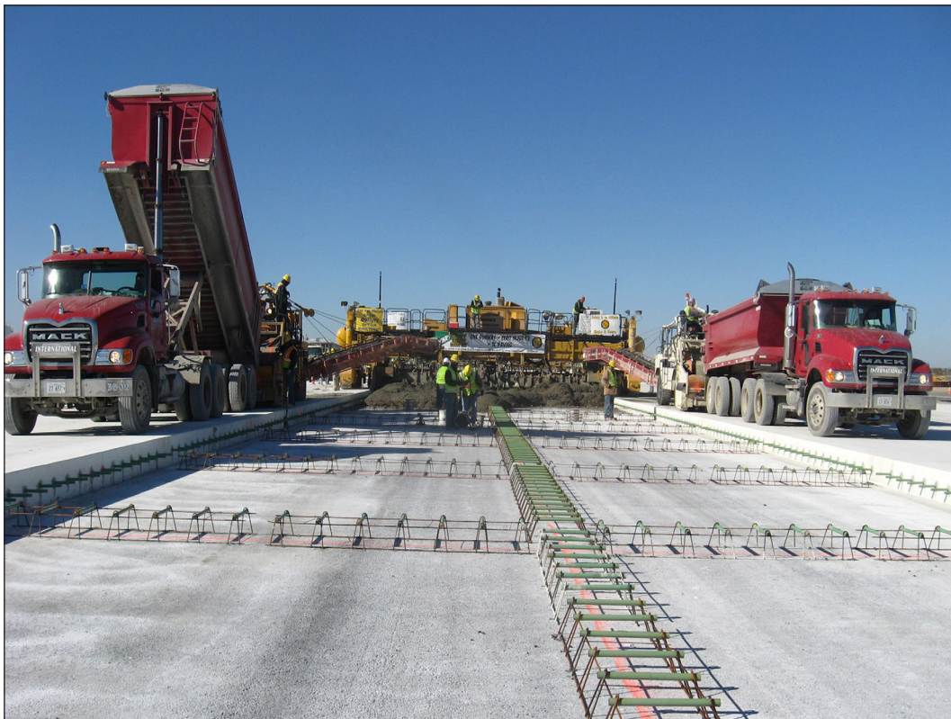
The O'Hare Modernization Program deeply entrenched in construction (photo courtesy of the Chicago Department of Aviation).
