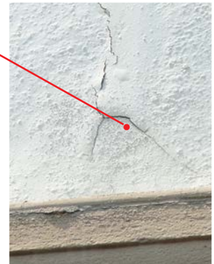
SUSPECTED WATER DAMAGE OF CEMENT PLASTER
