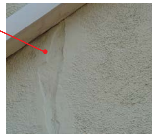
POOR CRACK REPAIR
