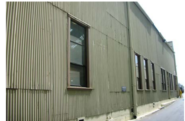
CORRUGATED METAL SIDING INDICATING PATCHING - AVENUE 12
