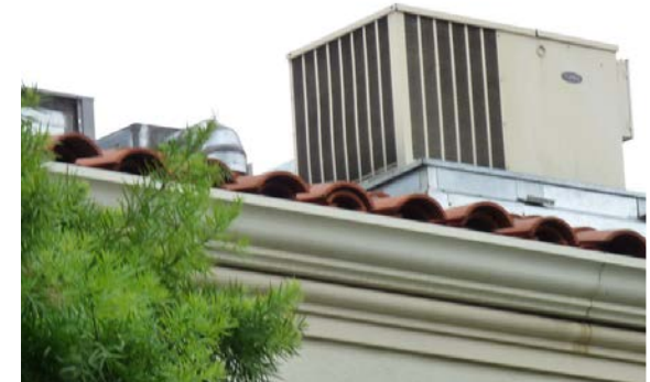
EXPOSED ROOF TOP EQUIPMENT
