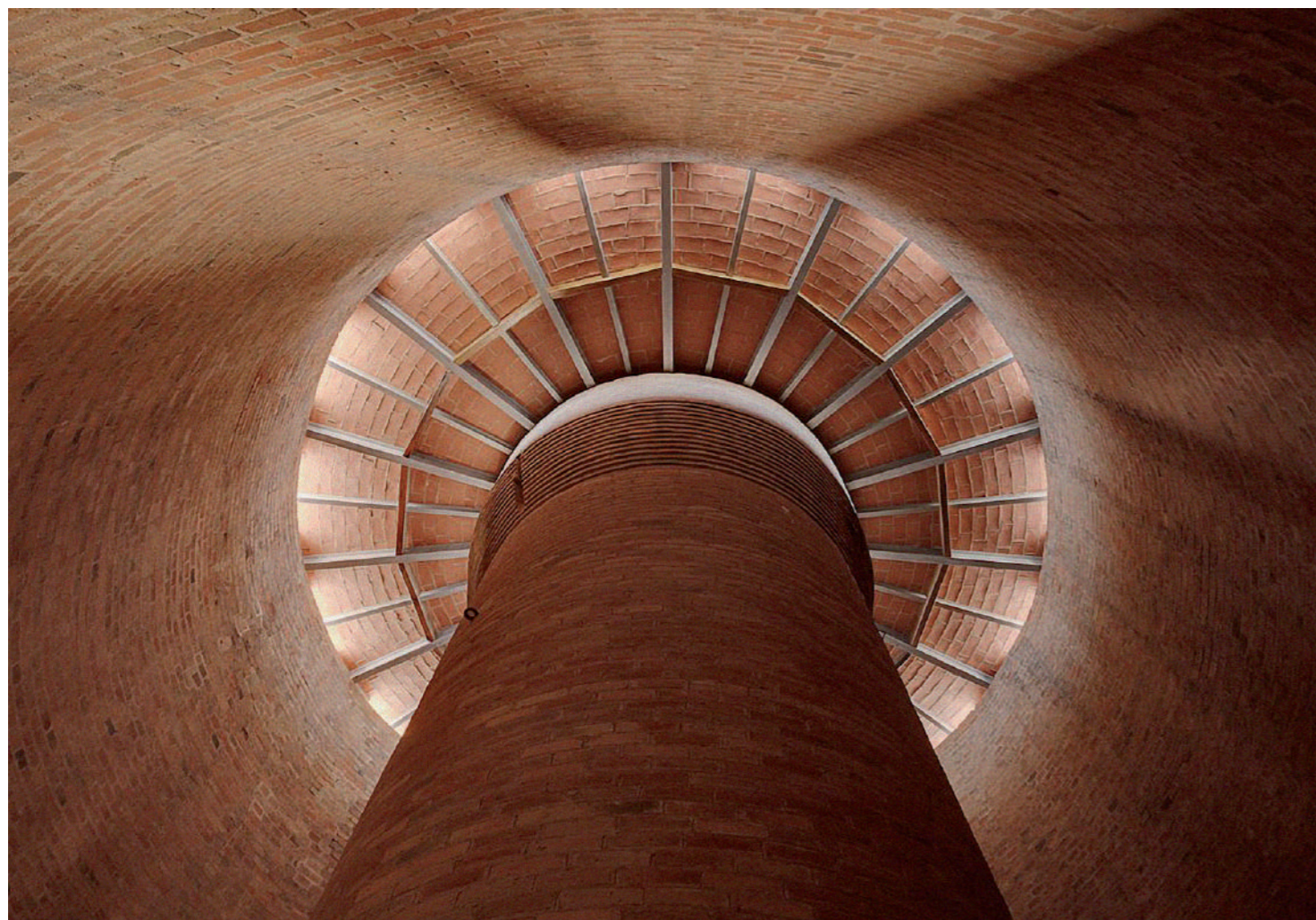
Pere Falqués's masterful use of the Catalan flat-brick timber vault technique creates interior spaces of striking elegance
