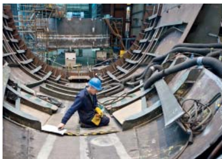
Platforms: Production of the Royal Navy's Astute-class nuclear-powered submarines continues, with the second of class, Ambush, undertaking commissioning, and boats three, four and five under construction.
