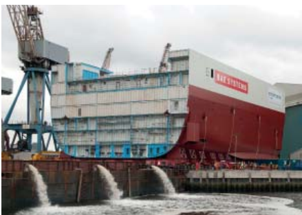
Platforms: Major block assemblies are in-build for the Royal Navy's new Queen Elizabeth class aircraft carriers.
