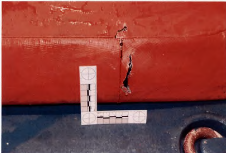
Figure 1.4.24 – Close up view of damage to BK-18 left intake blank top edge.
