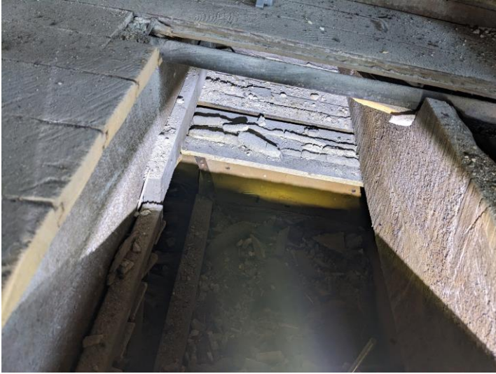
Image 16 – Second Floor – Damaged Joists Bearing on Modern Built Up 2x Wood Beam
