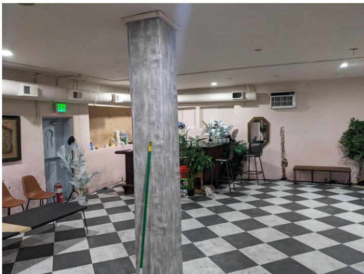
Image 20 – Main Level – Original Assumed Support Column for Original Assumed Steel Beam Above
