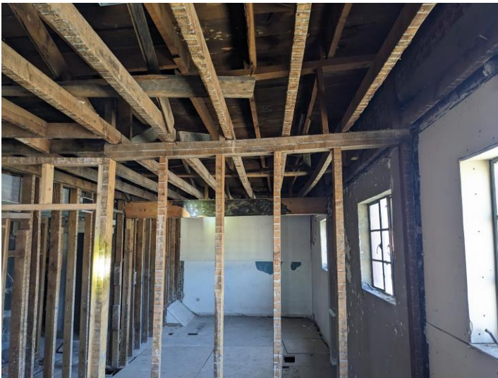
Image 13 – Altered Bearing Wall/Beam
