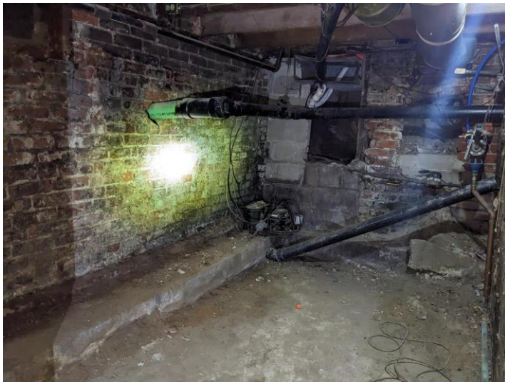
Image 26 – Crawl Space – Compromised Section – Northeast Corner
