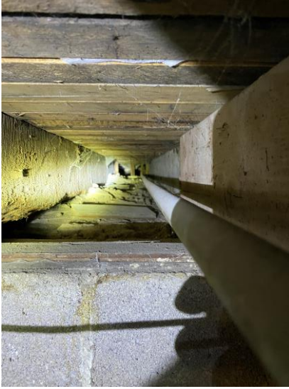
Image 22 – Main Level Framing – Existing Joists Above Soil
