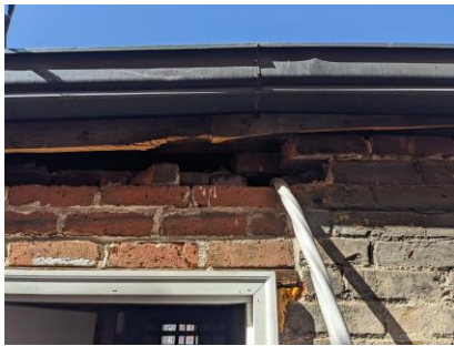
Image 7 – East Elevation – Top of Wall Deterioration
