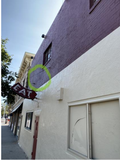
Image 6 – North Elevation – Area Where Wall Appears to be Bowing
