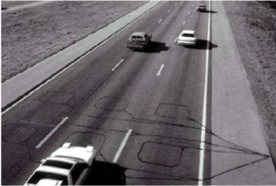
Figure 7: Typical Installation of Loop Detectors
