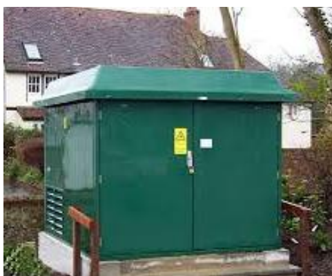
Figure 11: GRP substation enclosure
