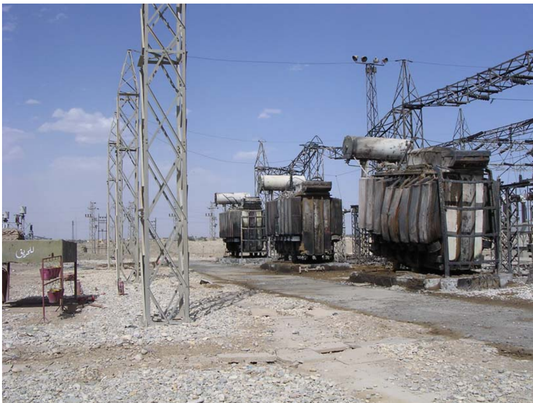
The United States attacked al-Nasiriyya 400 kV Electrical Power Transformer Station on March 22, 2003, with a carbon fiber bomb designed to disable power. The city lost power for thirty days. © 2003 Reuben E. Brigety, II / Human Rights Watch
