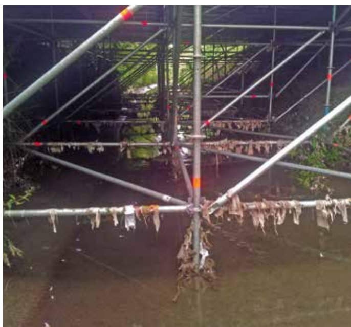
Figure 4.1 – Sewage related debris on scaffolding over the Blackstaff River
